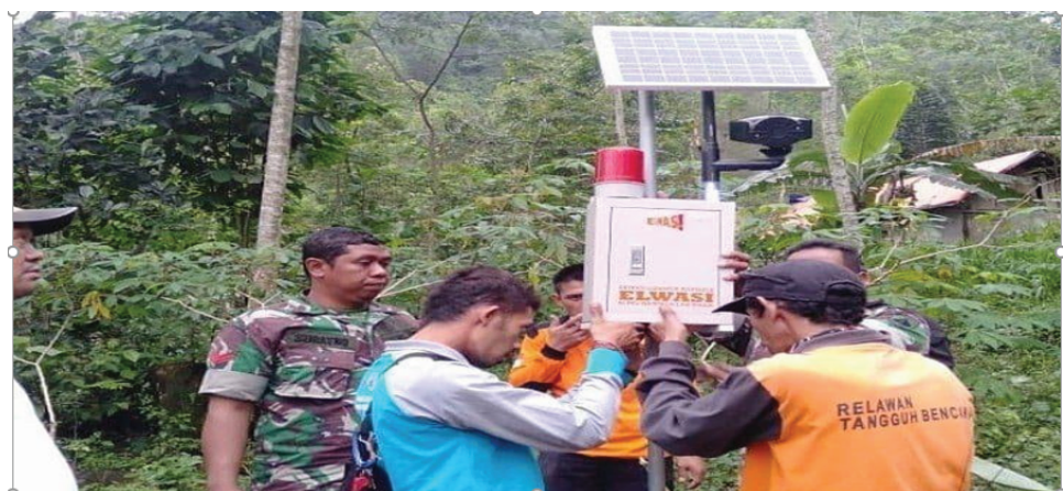
Figure 3: Installation of the Early Warning System (EWS) by BPBD Banjarnegara Regency. Source: BPBD Banjarnegara Regency, 2020.
