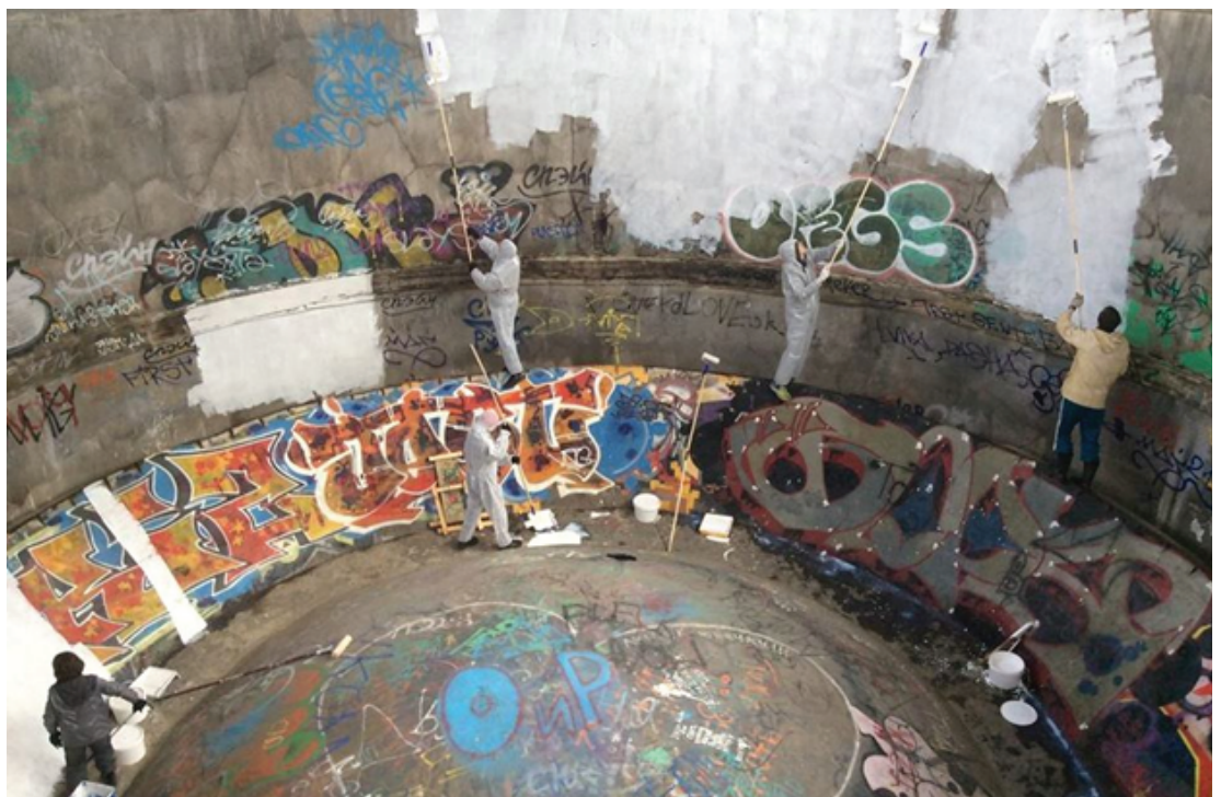
Figure 3: Working-party 2016. Work inside the tank. Preparation of walls as a screen for multimedia exposure. Podelniki’s public archive in the group in Facebook.
