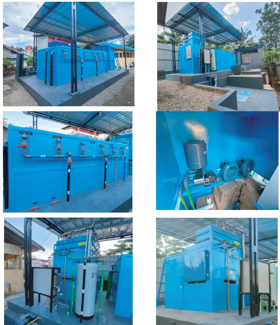
Figure 1: WWTP from Bhayangkara Hospital Kendari.
