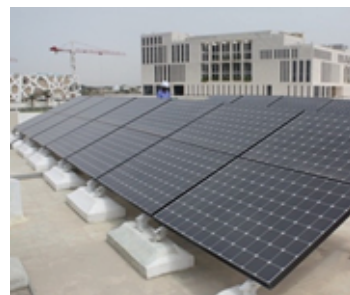
Figure 9: The roof-mounted PV system with ballasted racking on the roof.
