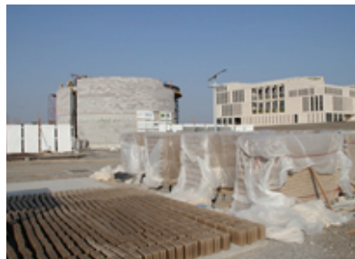
Figure 10: Production yard for compressed earth blocks set up on campus next to the EcoHaus site.
