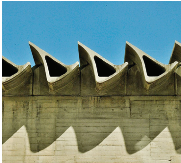
Figure 2: Detail of the “beams-bone” of the Center for Hydrographic Studies in Madrid.
