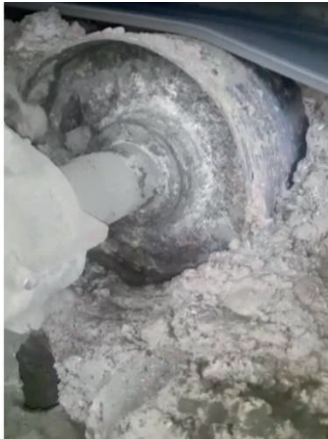
Figure 1: Case Material plug up in Weight Bridge of finish mill.
