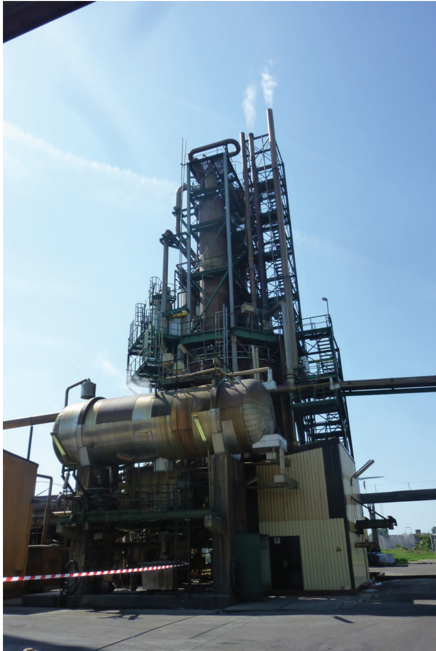
Figure 5: Gas treatment facilities of silicon carbide production in the company ESD-SiC (Holland).
