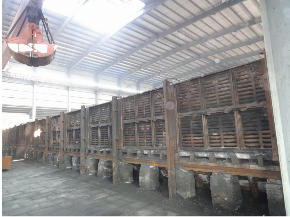
Figure 3: Stationary furnace 12 MVA in Xinjiang province (China).
