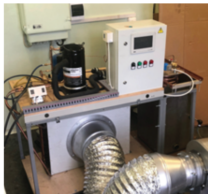
Figure 5: Heat pump unit for convective drying process.
