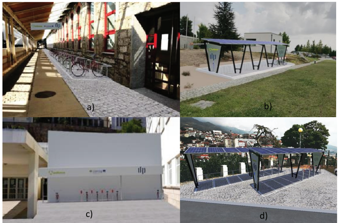
Figure 1: Charging stations installed in different spaces of the University of Beira Interior
