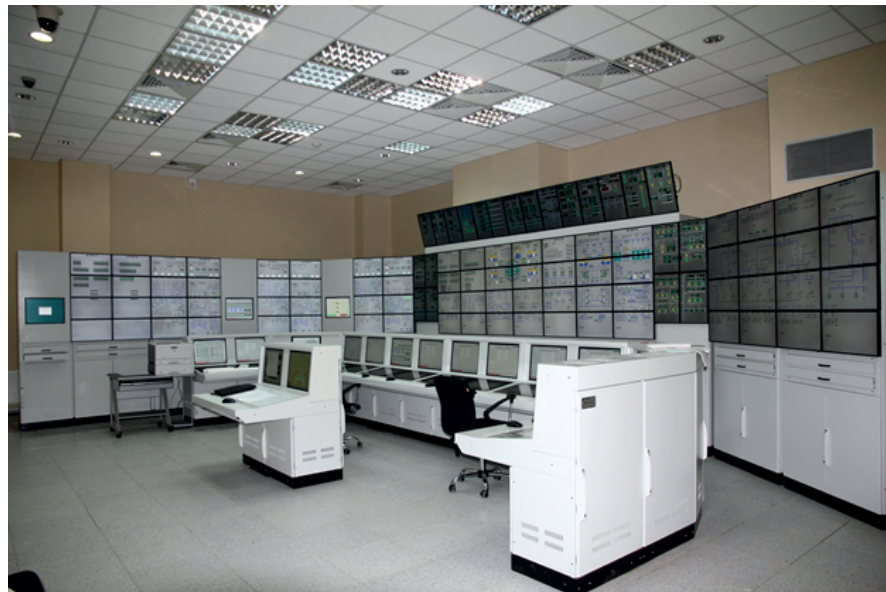
Figure 6: Analytical simulator of reserve control room of Kalininskaya NPP unit 4.
